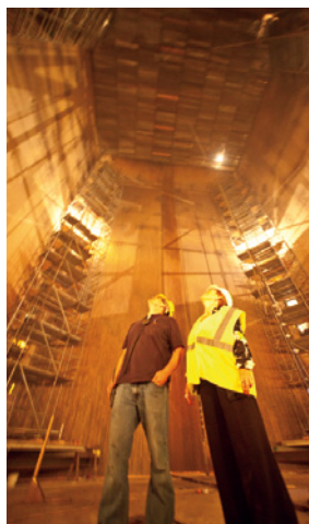
Madelen Schuemann, right, thermal operations manager, inspects the Boswell Unit 4 boiler with a contractor.
