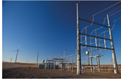
This new substation, built in 2010, serves the Bison Wind Energy Center.
