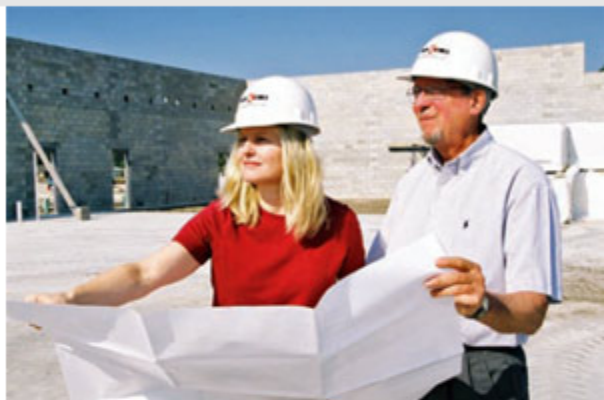
Laura Holquist, president of ALLETE Properties, and Bill Livingston, president of Palm Coast Holdings, at the Town Center construction site.
