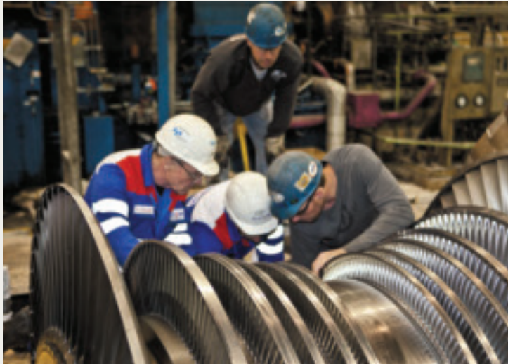
Millwrights from Lakehead Constructors and Minnesota Power workers inspect a new turbine rotor at the heart of a major rebuild of Boswell's Unit 4 generator.
