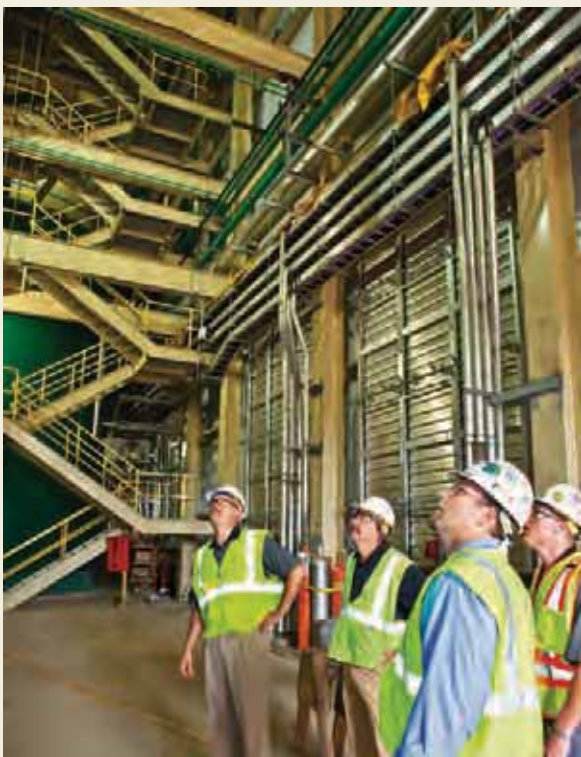
ALLETE President Al Hodnik, left, and others check out improvements at Boswell Unit 3, a major environmental retrofit completed in November of 2009.
